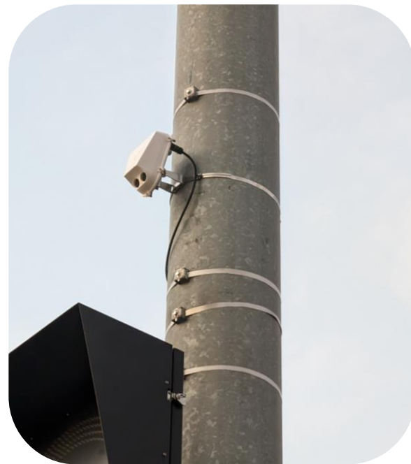
Sensor installed at Culver/Main
