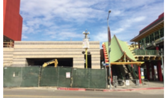
Sidewalk access is blocked for a construction project, forcing pedestrians into the street or to use less direct paths to the Metro facility.
